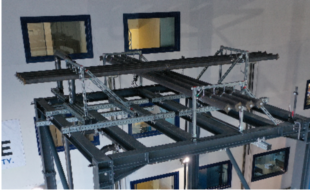
Figure 2.8: Pipe rack on the third floor
